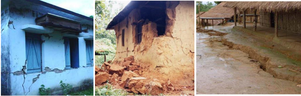
Figure 2: Building damages and ground displacement in Rangamati Earthquake in 2003 (image courtesy: www.cuet.ac.bd/ieer )
