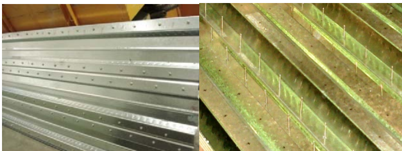
Figure 3: Steel deck with screws drilled from the bottom side (left) and a view from the top side (right)
