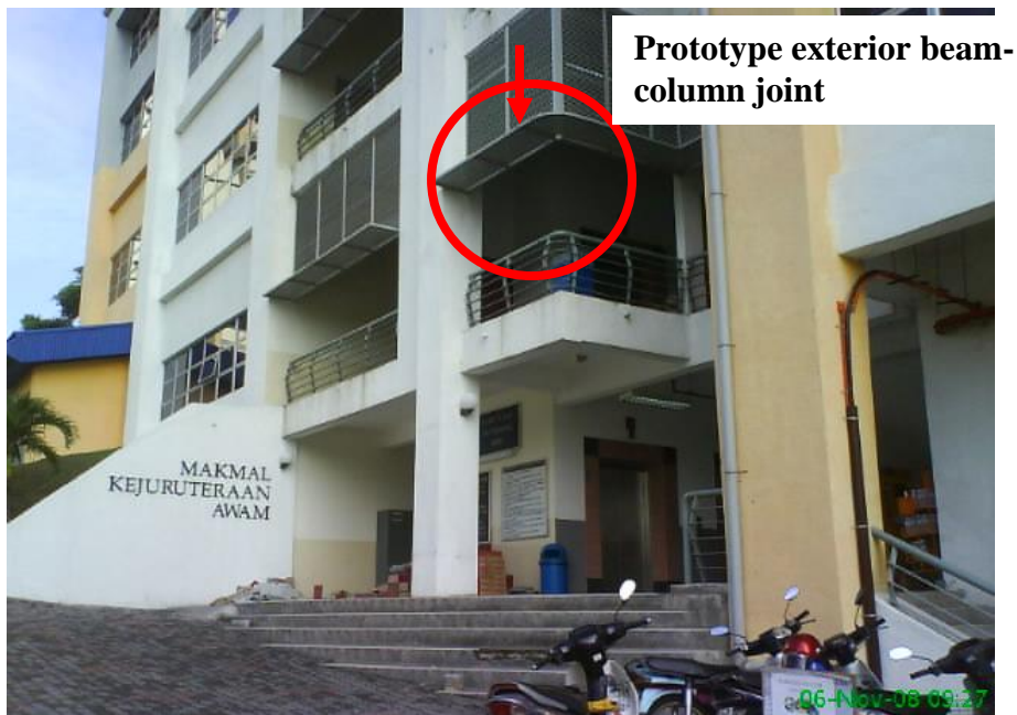
Figure 4: A prototype of exterior beam-column joint of ground floor of Block 1, Faculty of Civil Engineering, Universiti Teknologi MARA, Shah Alam, Selangor.
