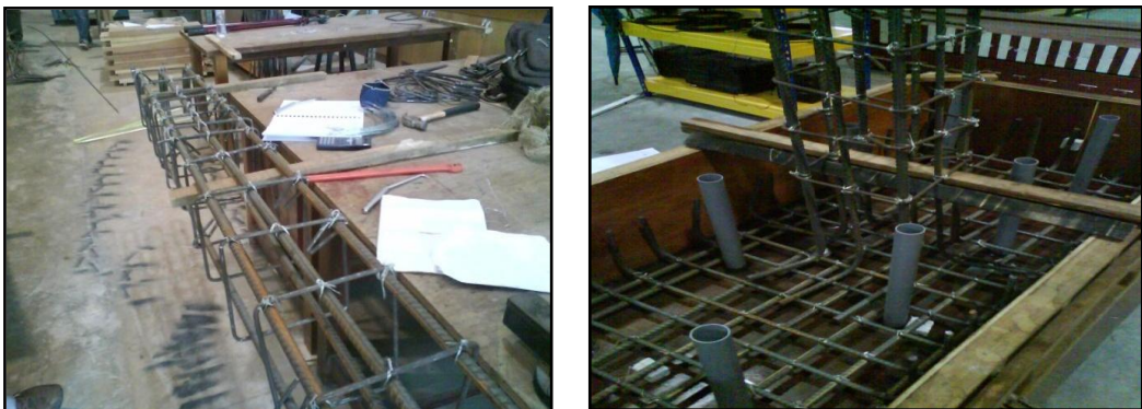
Figure 9: Construction of beam-column connection; (a) schematic arrangement of links in beam; and (b) location of PVC pipes in foundation beam before pouring concrete.
