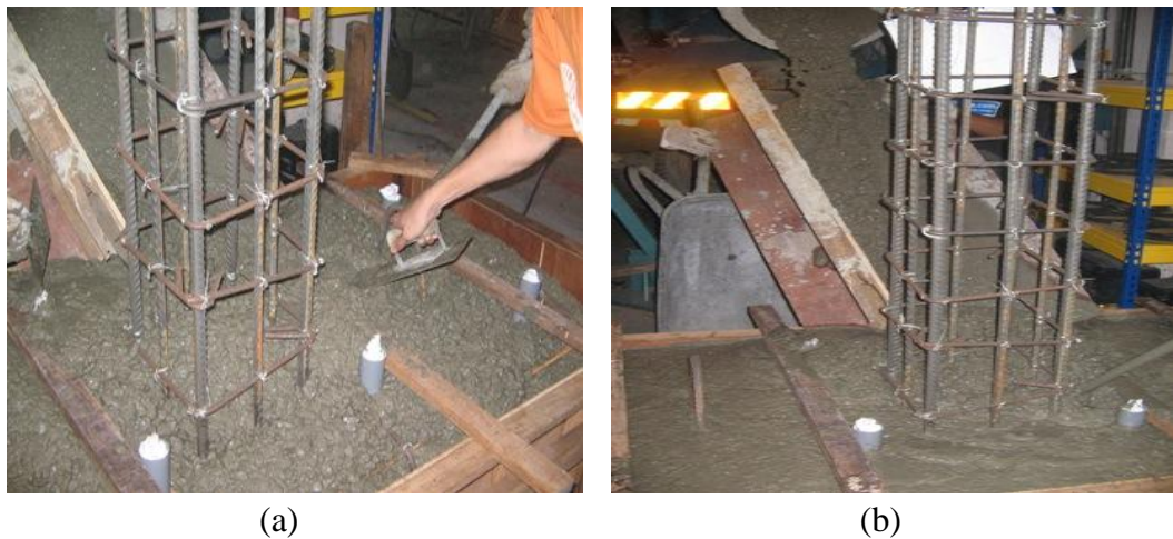
Figure 12: Process of concreting for foundation beam; (a) pouring concrete into the formwork of foundation beam; and (b) leveling top part of foundation beam up to PVC pipe.
