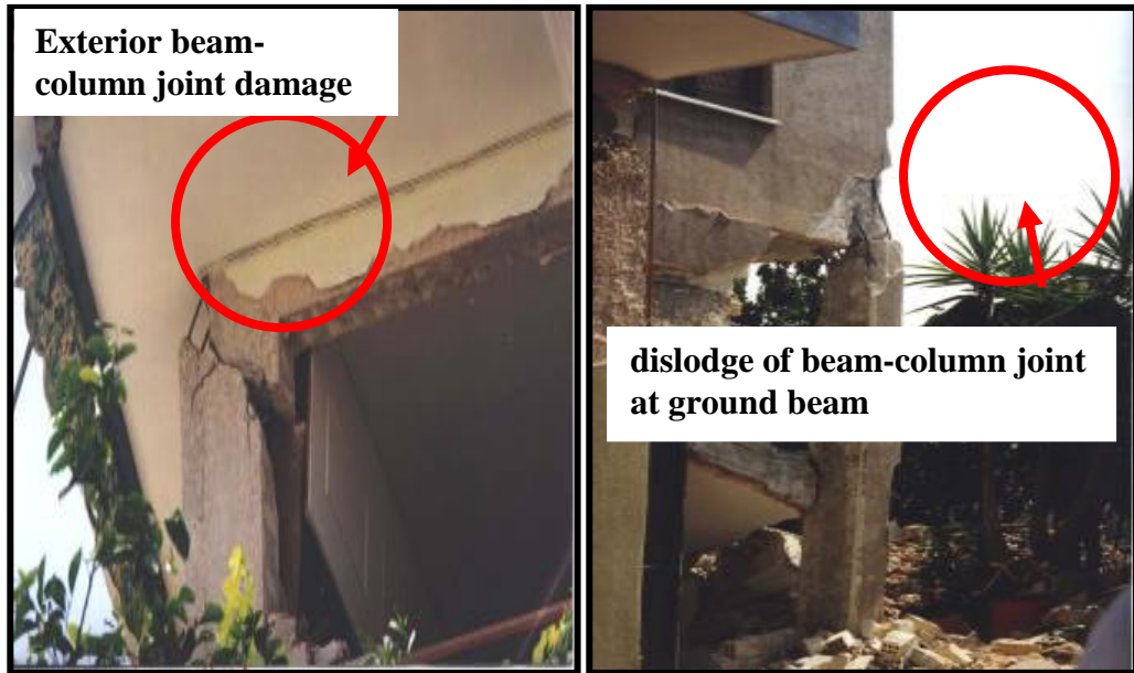
Figure 2: Beam-column joint damages during the 2001 Bhuj Earthquake India ; (a) Disorganization of a beam to column joint is inadequate; and (b) Overloading of exterior beam-column joints and lacking of stirrups.
