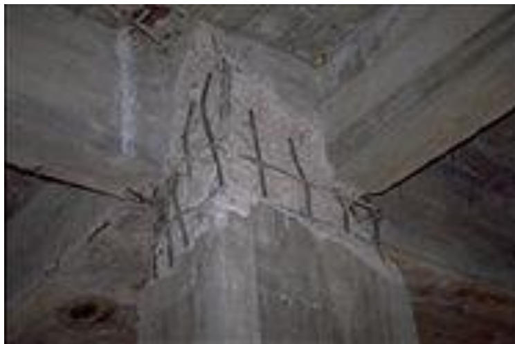
Figure 3: Spalling of concrete cover at beam-column joints in reinforced concrete building.
