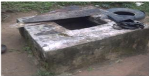
Figure 5: Sampled concreted shallow well with covered stained with bitumen
