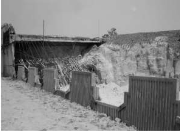
Figure 2 Failure of the RE wall at National Highway, NH-6 near Kolkata, India (A.Sengupta, 2012)
