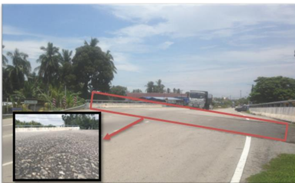
Figure 3 Settlement problem in Jambatan Parit Jamil
