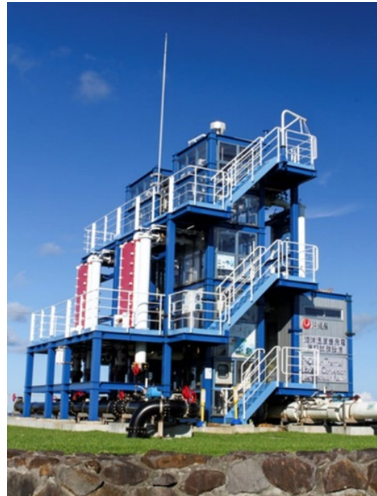
Figure 2 Okinawa Prefecture deep sea water ocean thermal energy conversion (OTEC) demonstration facility. (Source: OTEC Okinawa).
