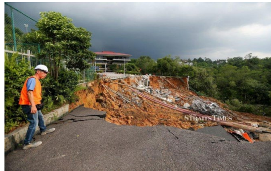
Figure 16 Landslide in front of MACA building, Kuala Lumpur
