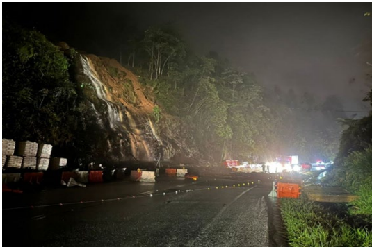
Figure 18 Landslide at Jalan Simpang Pulai Valley, Ipoh
